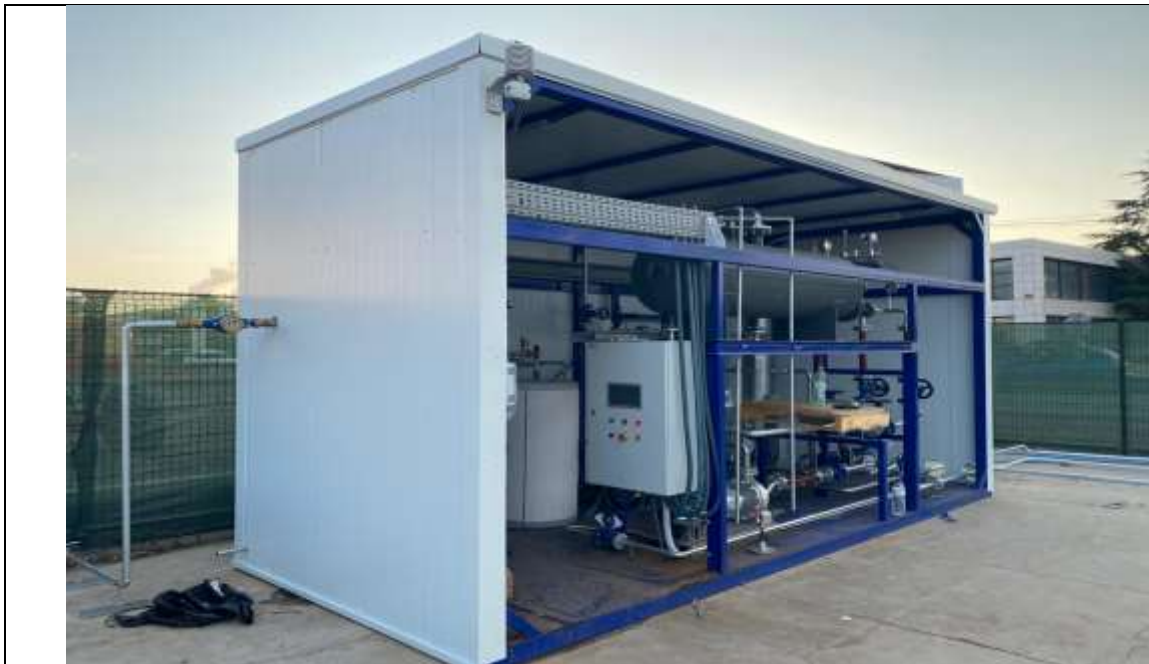
Figure 5. Skid developed by SOLATOM for the integration scheme shown in Figure 4.
