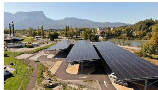
Ombrière la Chavanne 500 kWc – 2022 – Vente Totale -> autoconsommation collective
